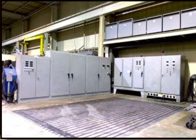
Flanders 6,900 volt test panel and isolation pad.
